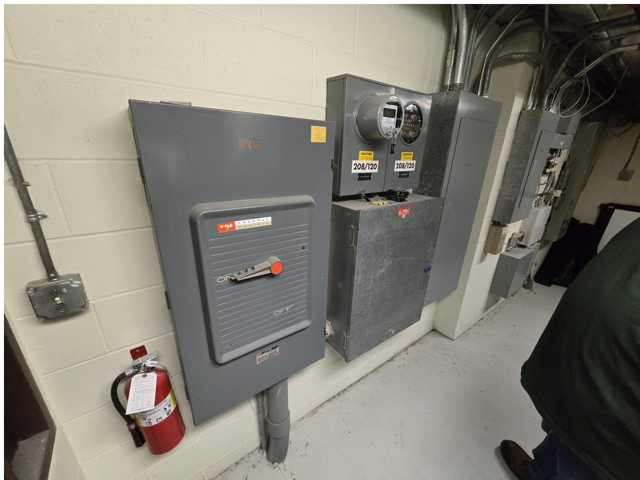
Outdated Electrical (Federal Pacific Electric went out of business in the 80's)
