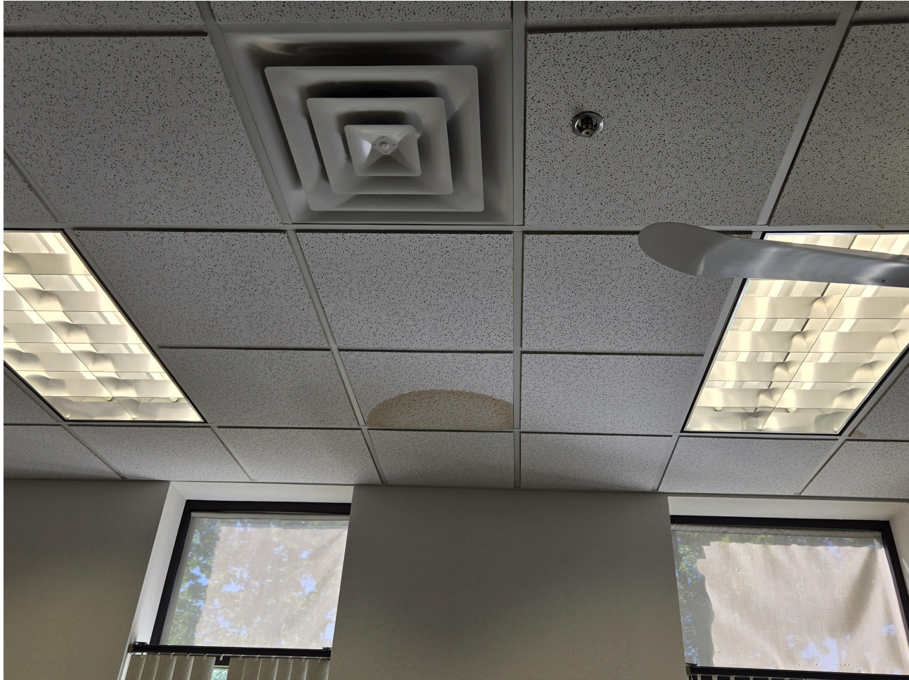
Ceiling damage (Ceiling tiles are due for replacement)
