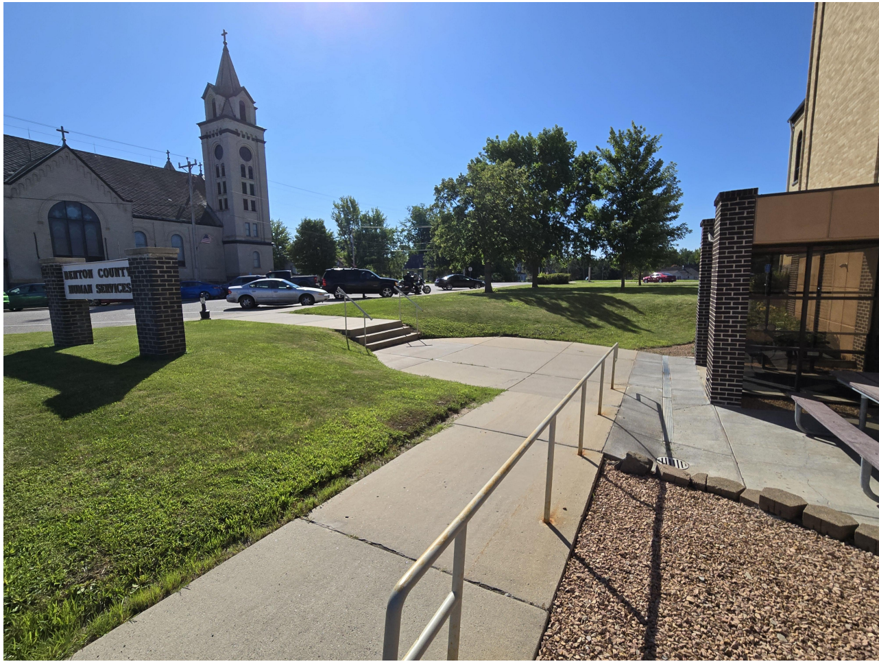
Improper drainage (water drains to building causing water damage/unsafe conditions)
