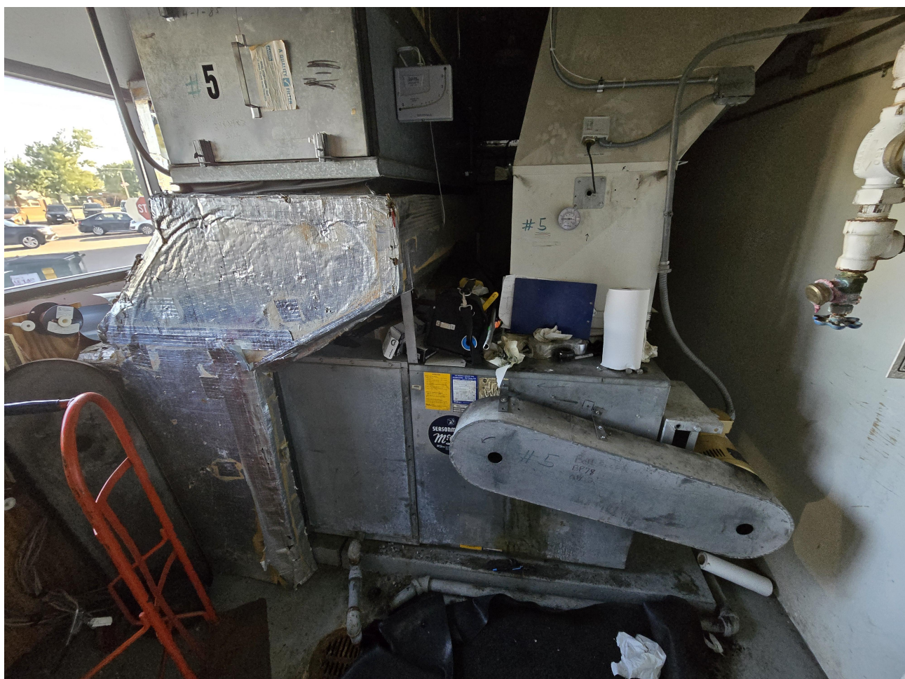
Outdated HVAC (HVAC systems due for replacement and old pneumatic style controls)
