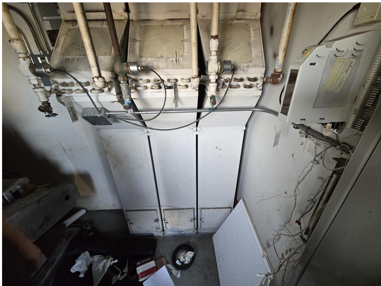
Outdated cooling (Inefficient, old style Freon, due for replacement)
