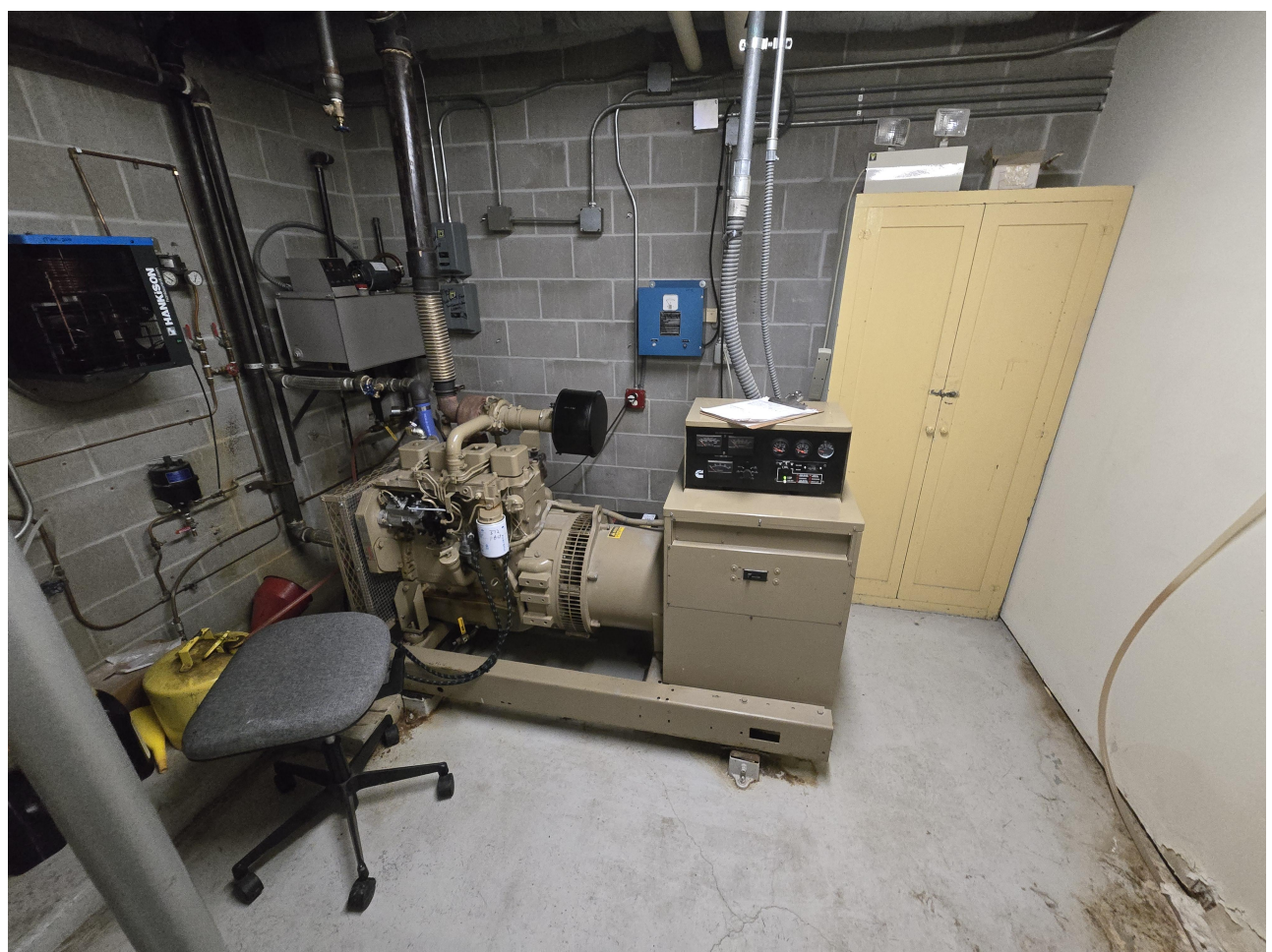
Undersized Generator (Minimal systems with backup power capabilities)
