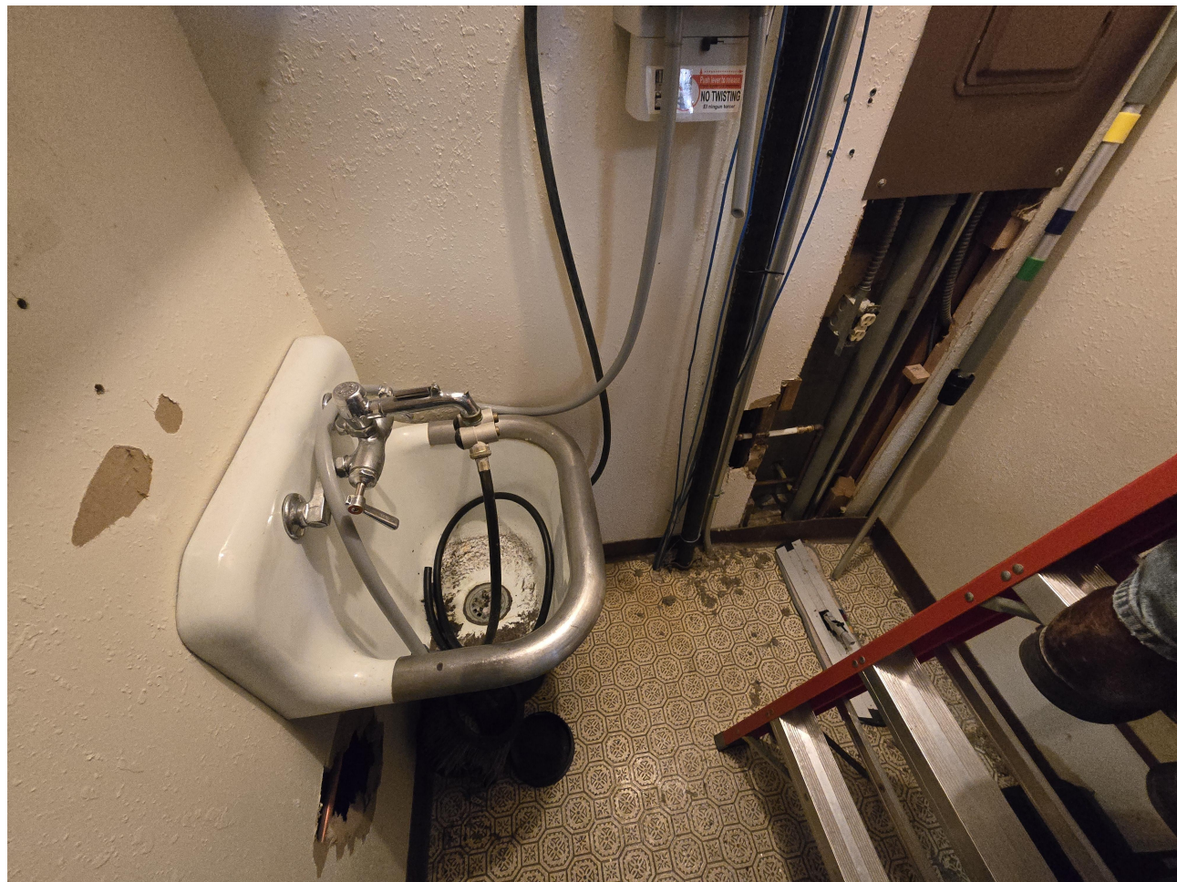
Utility room (Inadequate and aged supporting spaces)
