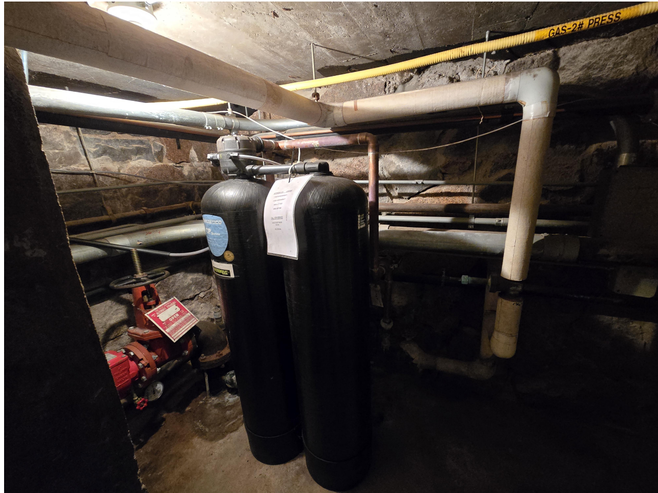
Sprinkler/water service (Basement location with inadequate space and clearance)
