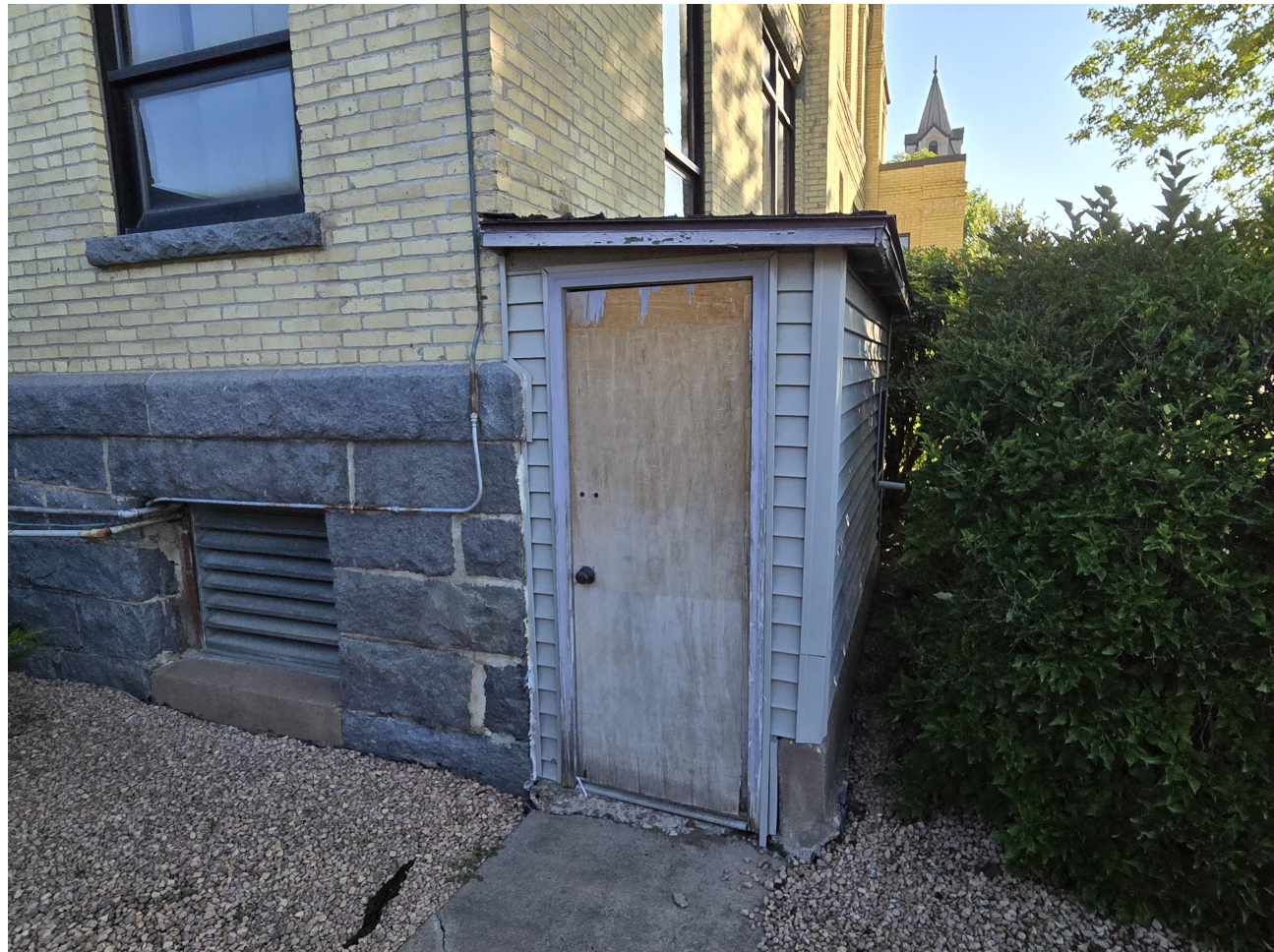
Exterior entrance (Needs replacement or removed for security)
