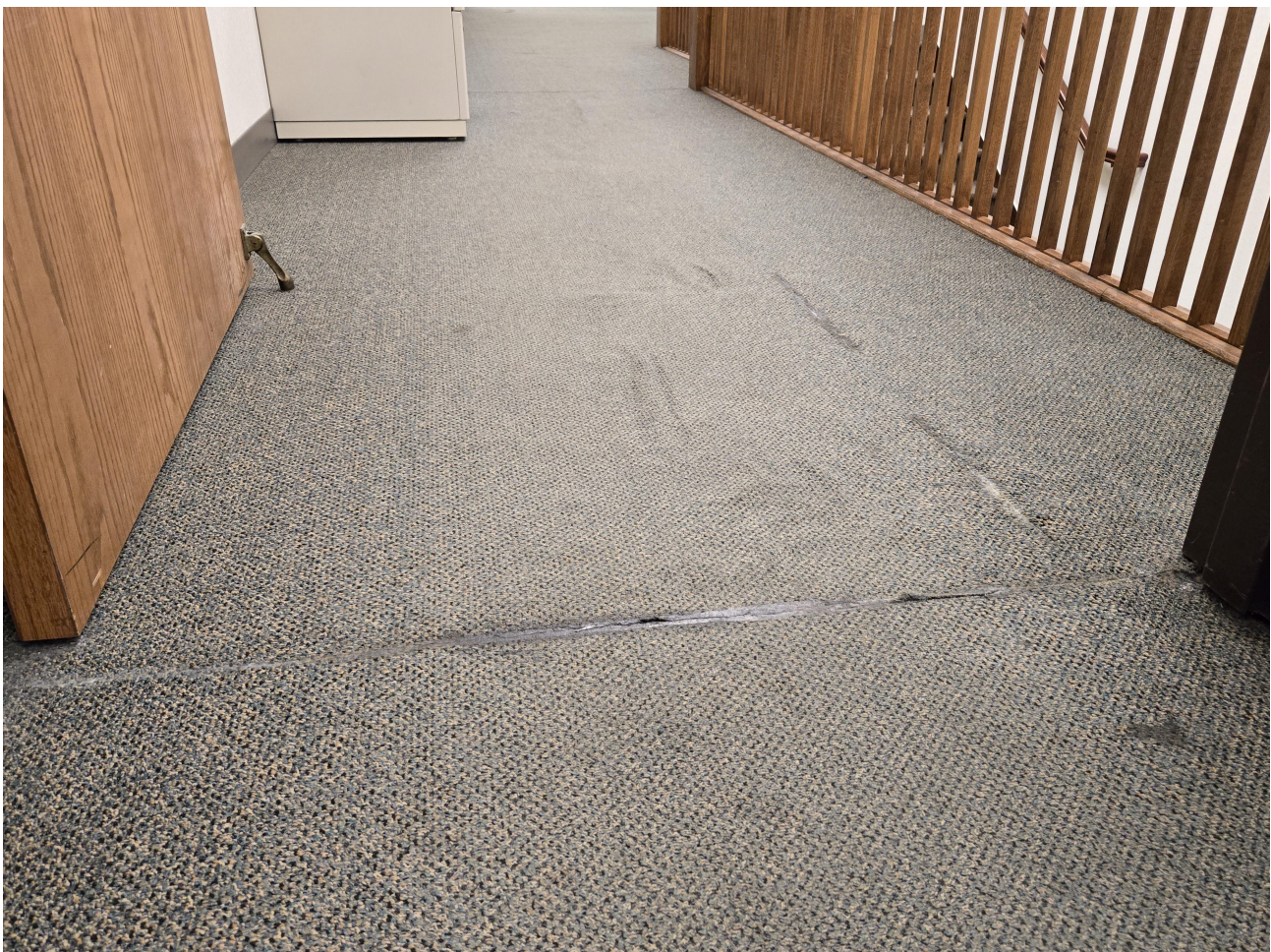
Worn out finishes (Carpet, doors, paint, etc. due for significant replacement)
