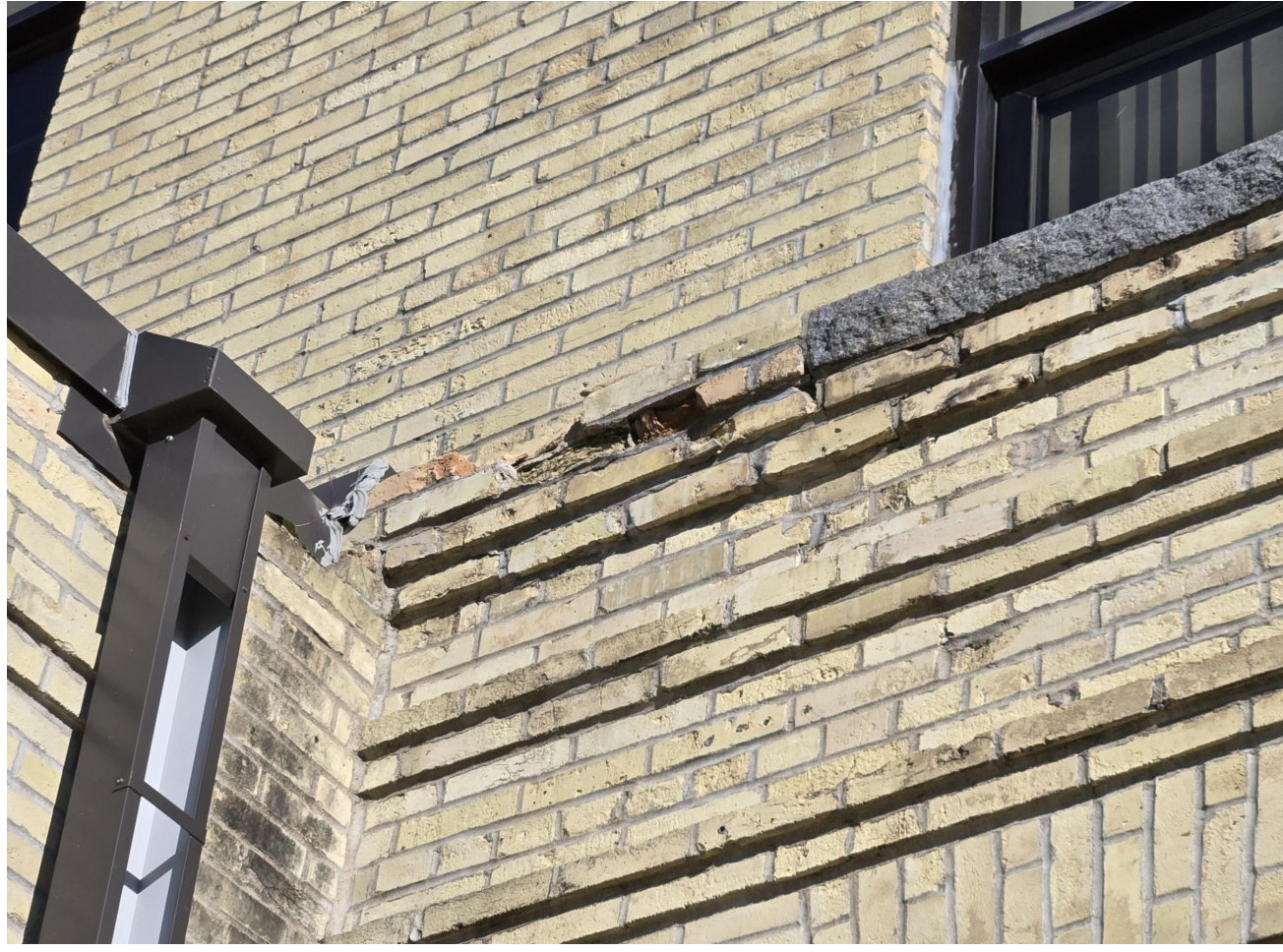
Masonry degradation (Brick spalling and water infiltration, brick replacement needed)
