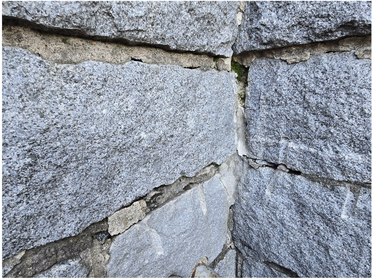
Tuck pointing and sealants (stone mortar and all exterior sealant due for replacement)
