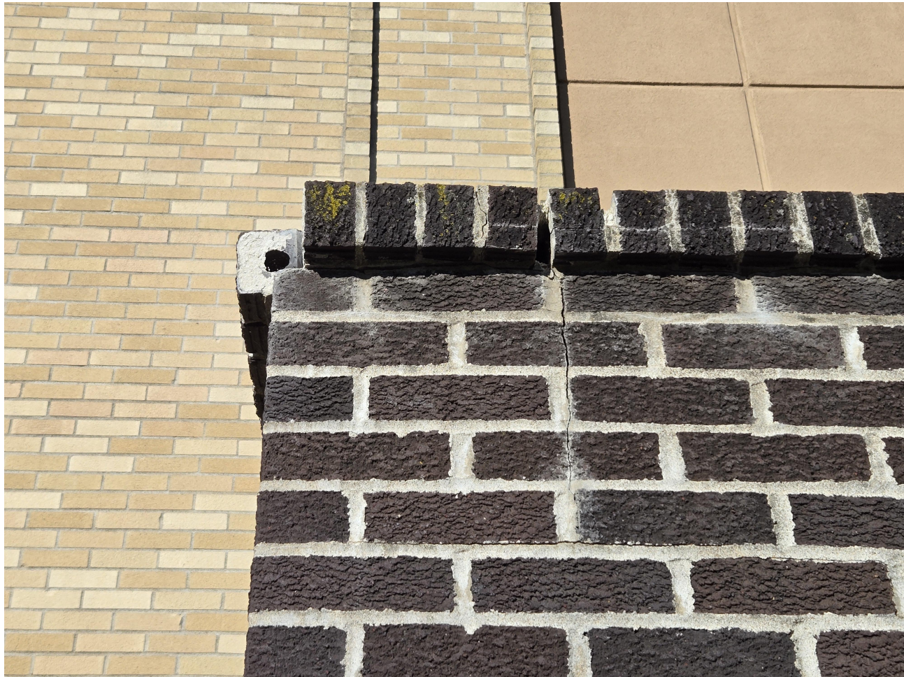
Masonry cracking (Brick and mortar repairs needed)
