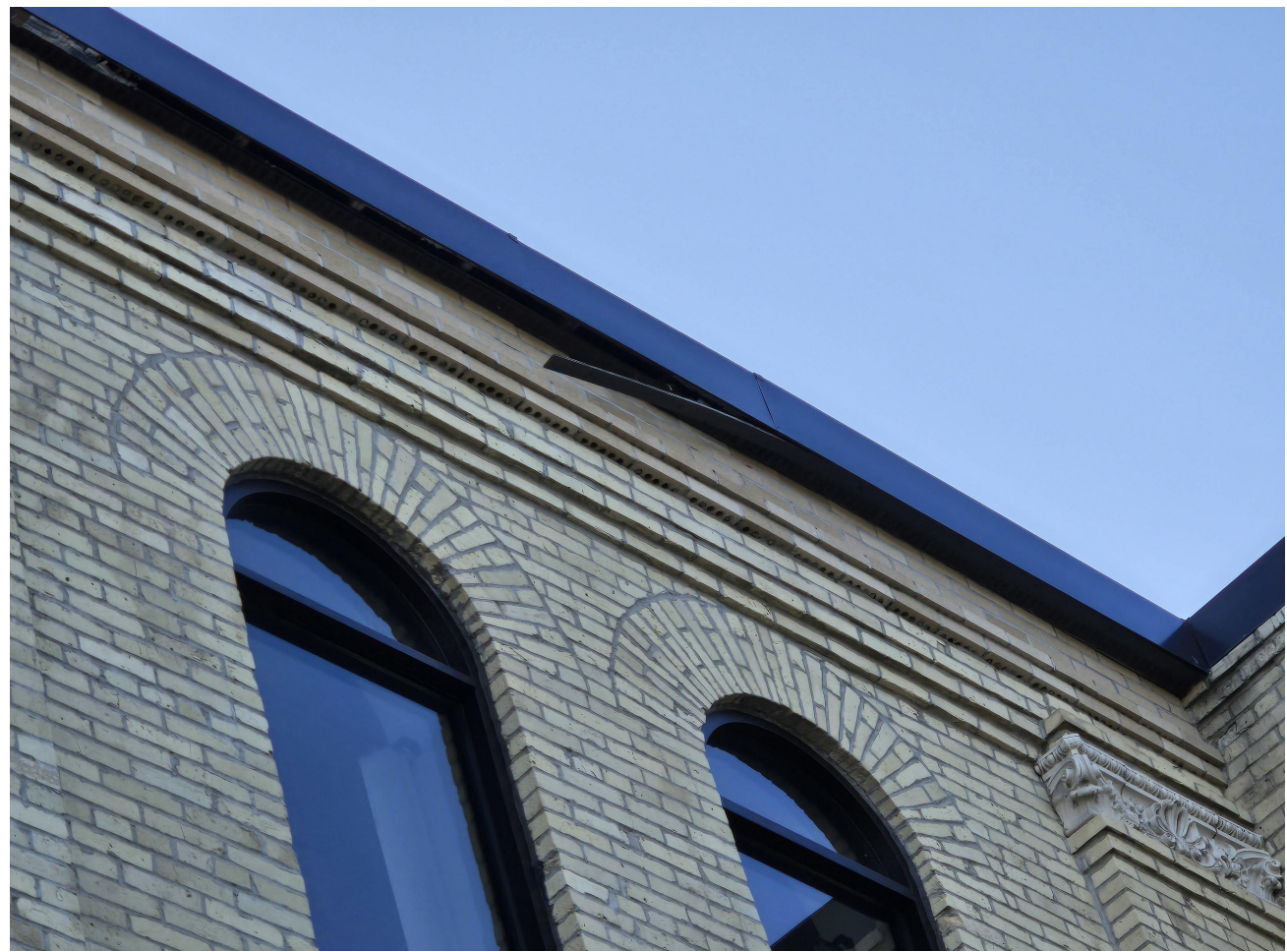
Flashing damage (Parapet area flashings need repair or replacement)
