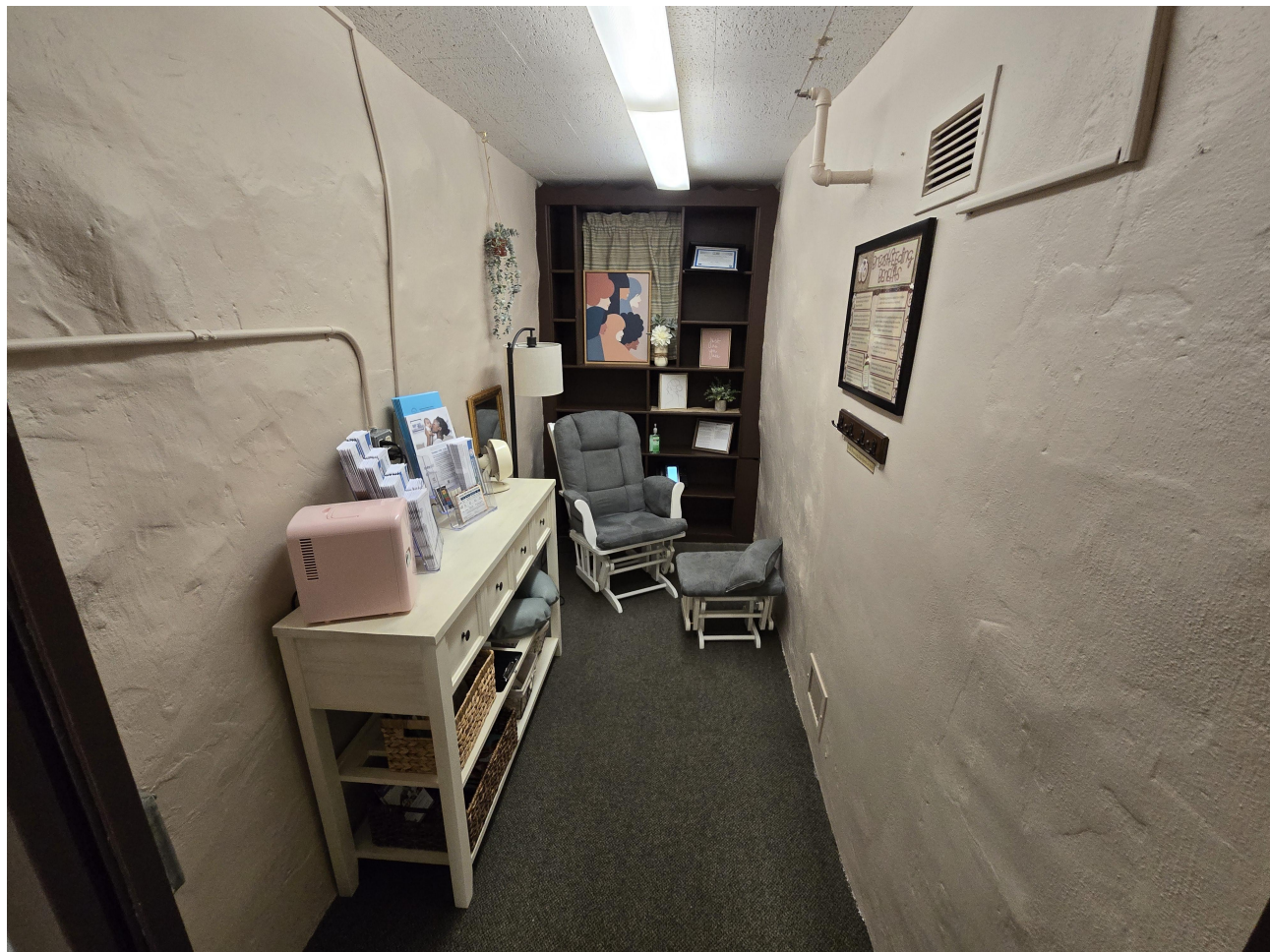
Difficult to remodel (Concrete walls and thick old exterior walls due to multiple additions)
